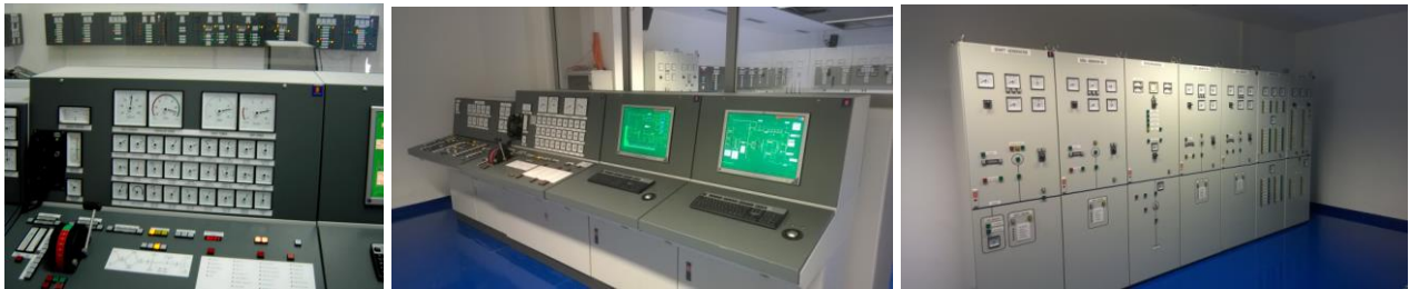
Kongsberg Engine Control Room (ECR)
